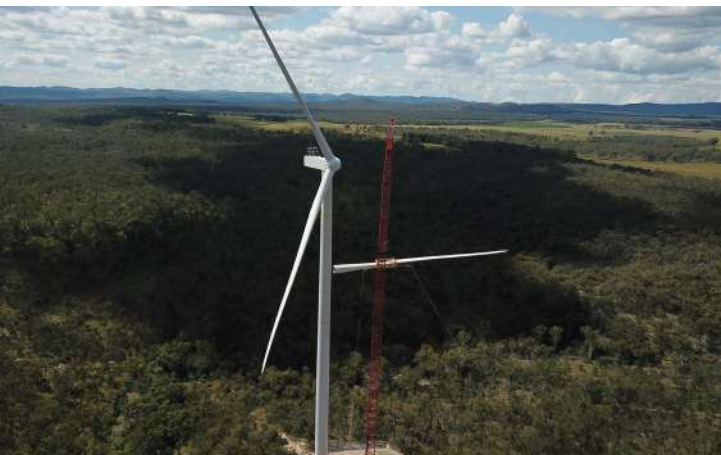
Mt Emerald Wind Farm. Image Courtesy: Queensland Government.
