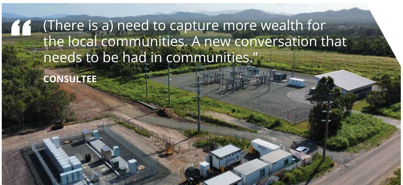
Tanby Battery. Image Courtesy: Energy Queensland.
