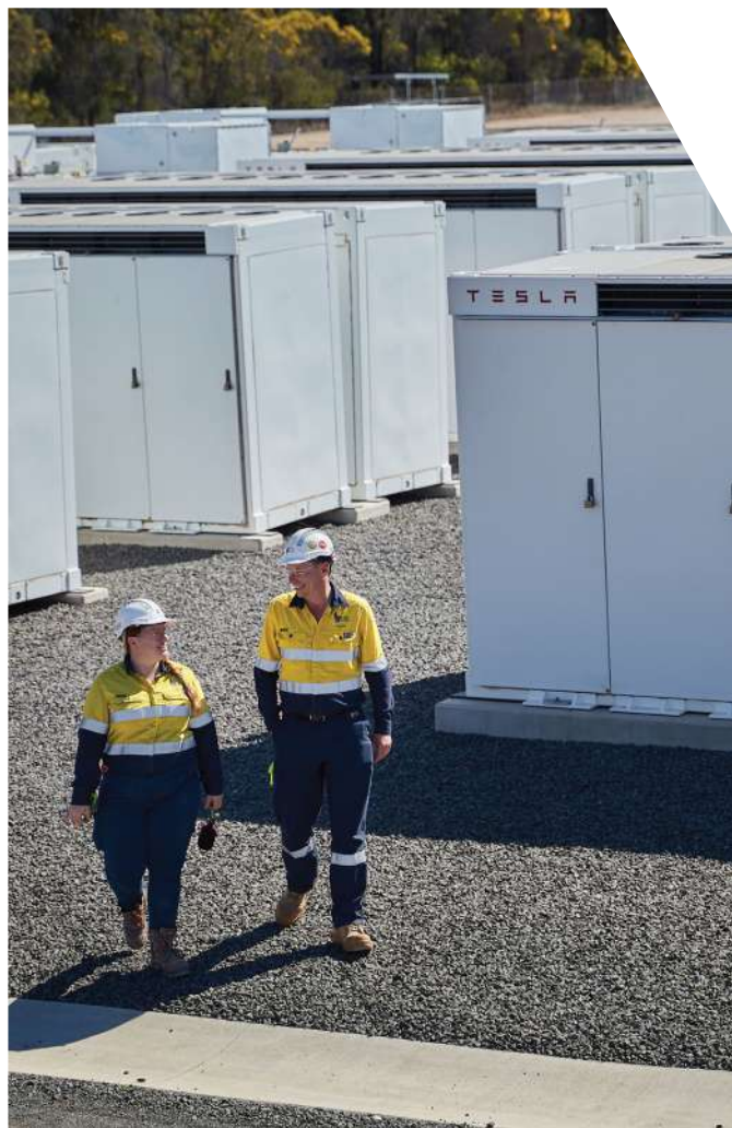
Chinchilla Battery. Image Courtesy: CS Energy.
