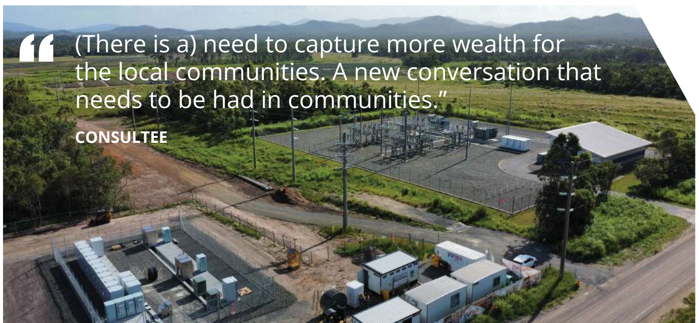
Tanby Battery. Image Courtesy: Energy Queensland.
