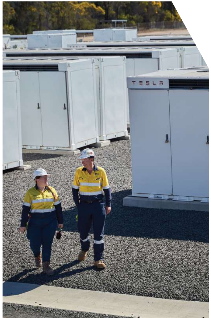
Chinchilla Battery. Image Courtesy: CS Energy.
