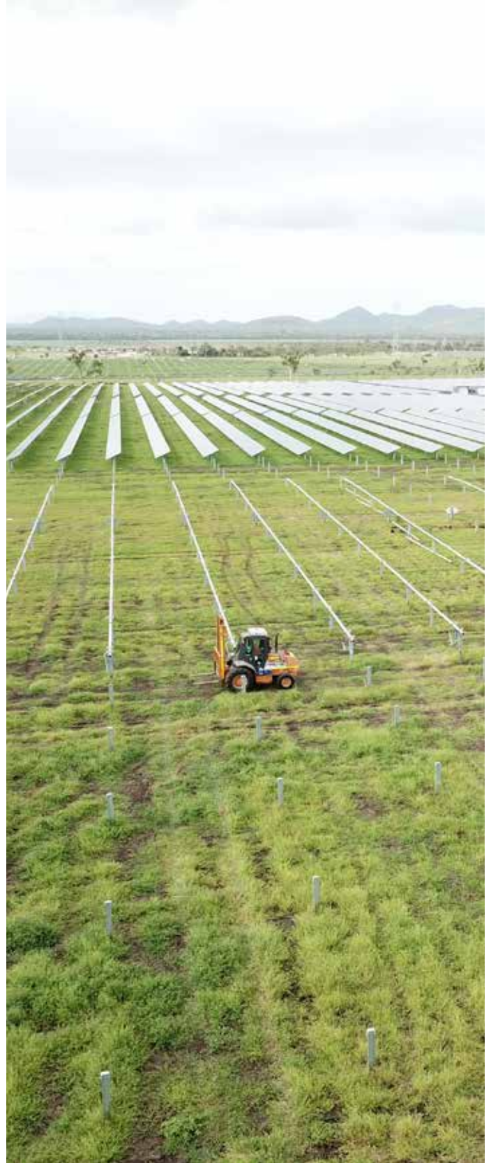
Whitsunday Solar Farm. Image Courtesy: Edify Energy
