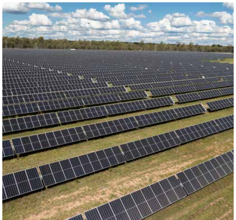
Western Downs Green Power Hub. Image Courtesy: Queensland Government
